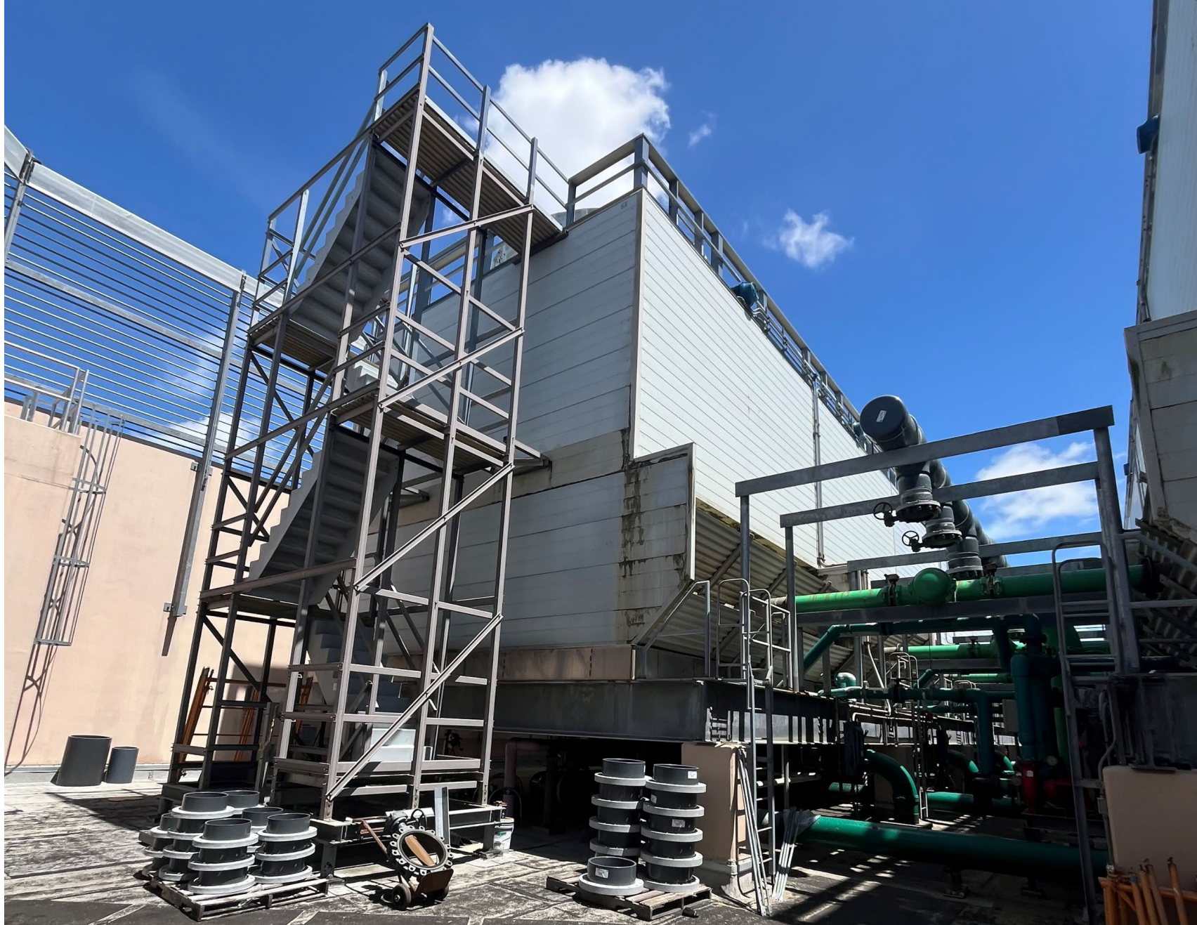
FEFPA 2024 Summer Conference Presentation: NSU Chiller Plant “Sharks on Ice” Design, Build, Operate and Maintain
