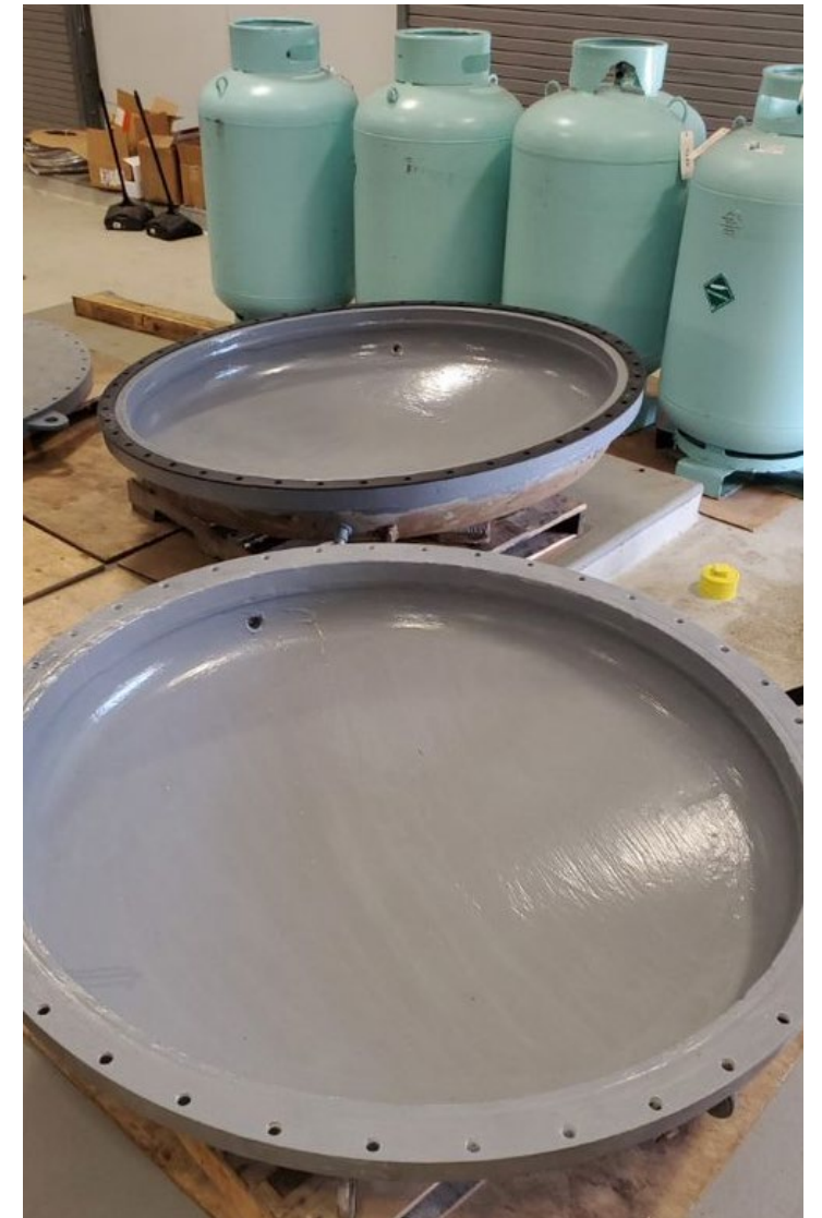
Chiller #2 End Bell Following New Epoxy
