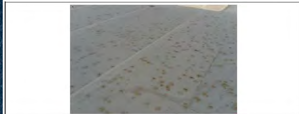
Fig. 3.1.1-1. Single-ply membrane roof 0.045 in. (1.1 mm) thick cut by hail
