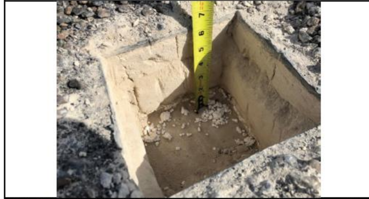
Photo 22: The depth of the roof assembly at Core #2 was approximately 6 1/4 inches. Based on the distance of approximately 50 feet between the two core samples, see Photo 20 , the slope is minimal at 1/4 inch within 50 feet.
