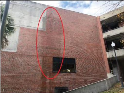
Photo 8: Overview photo of Test Area #2. The spray rack was positioned approximately 5 feet above the fourth-floor line and focused on the brick veneer approximately 6 feet adjacent to Test Area #1.
