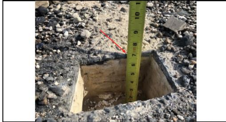
Photo 21: Core samples revealed the sloped roof substrate being a Zonolite LWIC material, over approximately 1 inch of Styrofoam insulation, Photo 29 . The depth of the roof assembly at Core #1 was approximately 6 1/4 inches.
