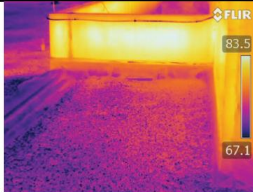
Photo 59: IR image at transition to the center area of the roof looking south along the parapet wall. The wall is showing high temperatures. While thermal anomalies are present, portions of the anomaly could be a result of reflectivity of the wall on the roof.
