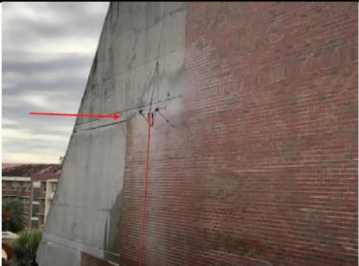
Photo 3: Approximately 1 hour into the test procedure, the spray rack was moved vertically approximately 10 feet and focused on the interface of the brick veneer to the poured in place concrete.
