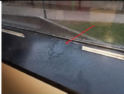
Photo 7: Water migrating from head condition and dripping on sill as a result of the test procedure.
