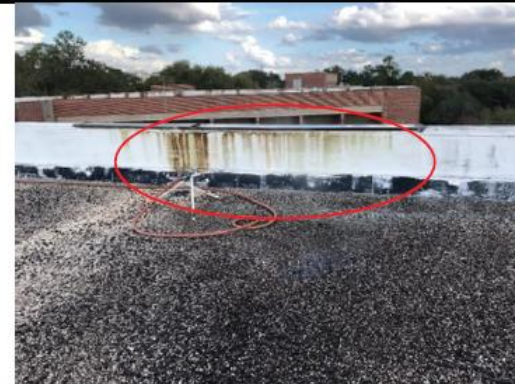
Photo 15: Overview photo of Test Area #3. Test Area #3 included the roof side of the parapet above Test Areas #1 & 2.
