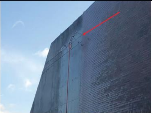
Photo 4: Approximately 3 hours into the test procedure, the spray rack was moved vertically approximately 10 feet and focused on the poured in place concrete. The vertical transition between the brick veneer and concrete was included in the test area.
