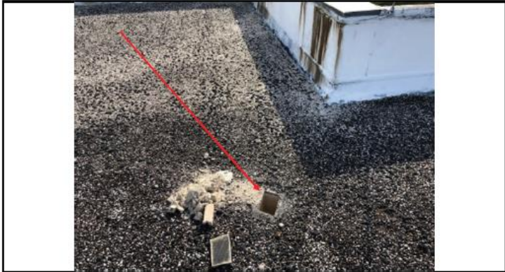
Photo 19: Photo to show general location of Core #1 at the south section of the East Wing roof area. See Photo 20 .
