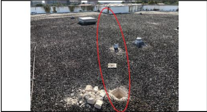
Photo 20: General location of core samples #1 and #2 at the East Wing roof area.
