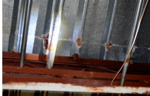
Rust on Connection Joists
