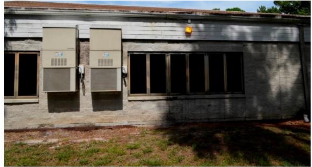
Typical Exterior Wall Pack with Damaged Mount
