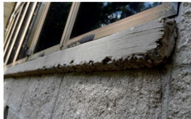
Cracks & Gaps at Windowsills & Poorly Cast Sill
