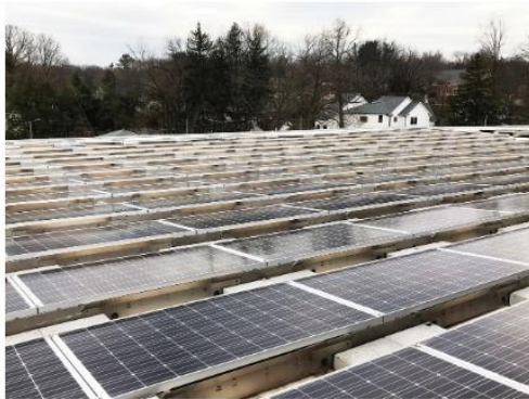
A view of the 1,700 solar panels on the roof of Discovery Elementary School in Arlington, Virginia. Over the course of the year, these panels provide more than enough energy to power the school.
