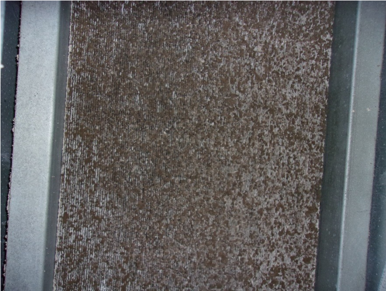
Reheat Coil - Before Remediation
