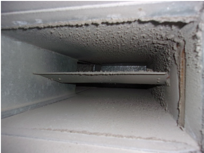
Ductwork - Before Remediation
