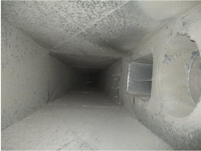
Ductwork - Before Remediation
