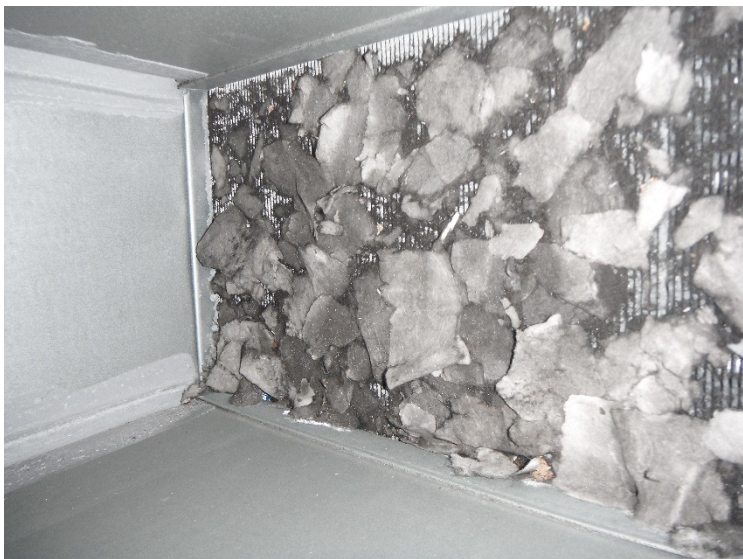
Reheat Coil - Before Remediation
