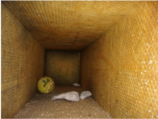
Ductwork - Before Remediation
